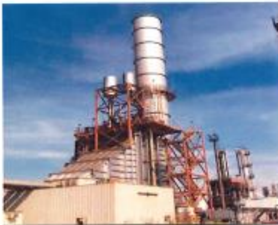
Turbina General Electric
